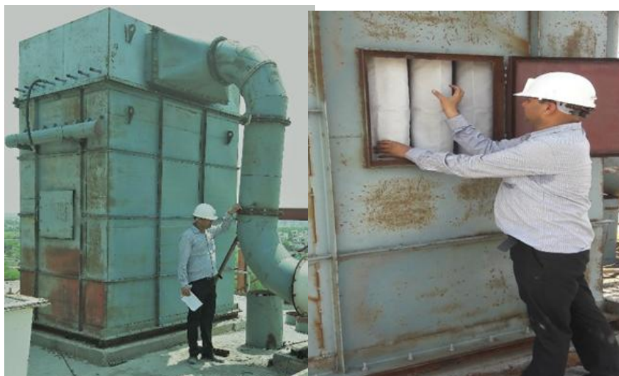
Fig. 3b Silo mounting, Target box Vent box with bag filters arrangement.
